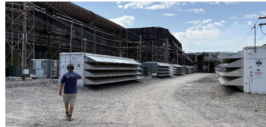
Above: Canaan's hosted miners in Midland, PA Operated by Mawson Infrastructure Group
